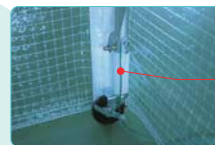
Pipe with ground terminal
